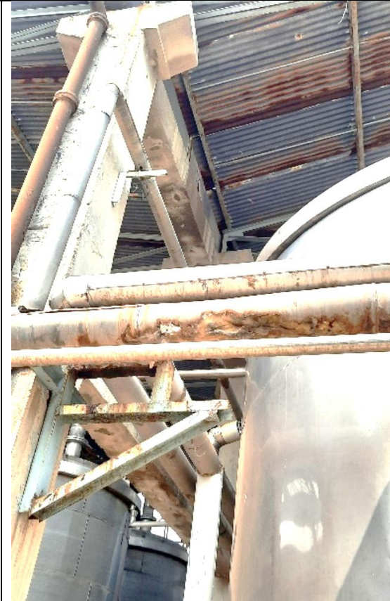
Rusted pipes up-stair on roof
