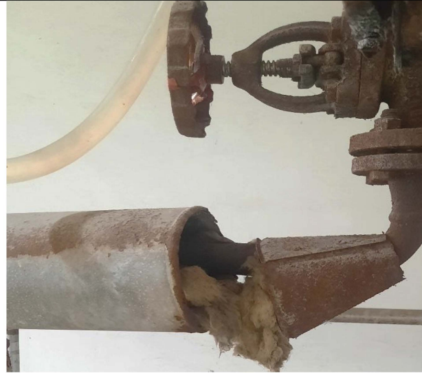
Improper maintenance of pipes by the contractor
